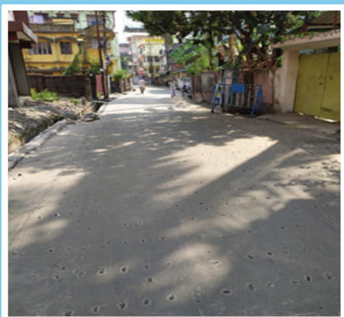
NAME OF WORK : Repairing and upgradation of APC Sarani 1from DBC road to PIPE line under Siliguri MC ESTIMATED AMOUNT : Rs. 62,51,105
