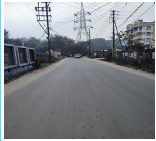
NAME OF WORK : Improvement of Bituminous road S/f PateshwarySchool to Don bosco Road at Ward no-41 ESTIMATED AMOUNT : Rs. 76,58,187
