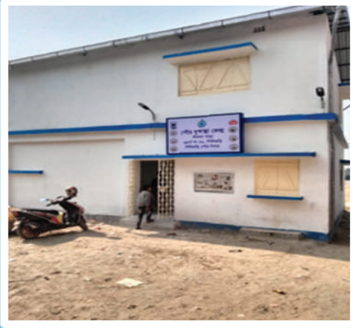
NAME OF WORK : Repairing and renovation of Sitlapara community hall at ward no 31 ESTIMATED AMOUNT : ₹ 13,80,060.00
