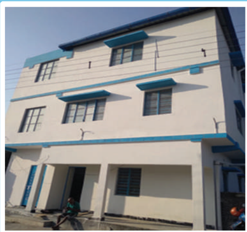
NAME OF WORK : Repairing and renovation of Prakash Nagar community hall at ward no 43.
